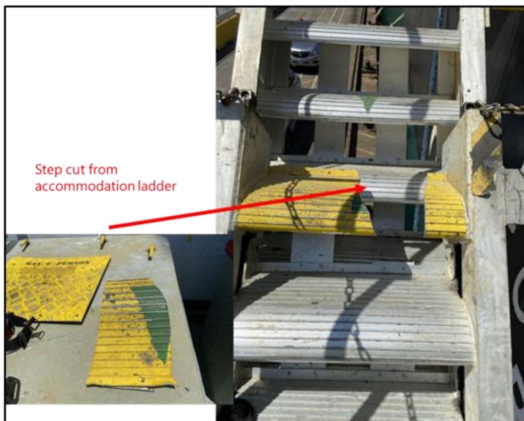
Figure 7: Step cut from the lower section of the ladder
