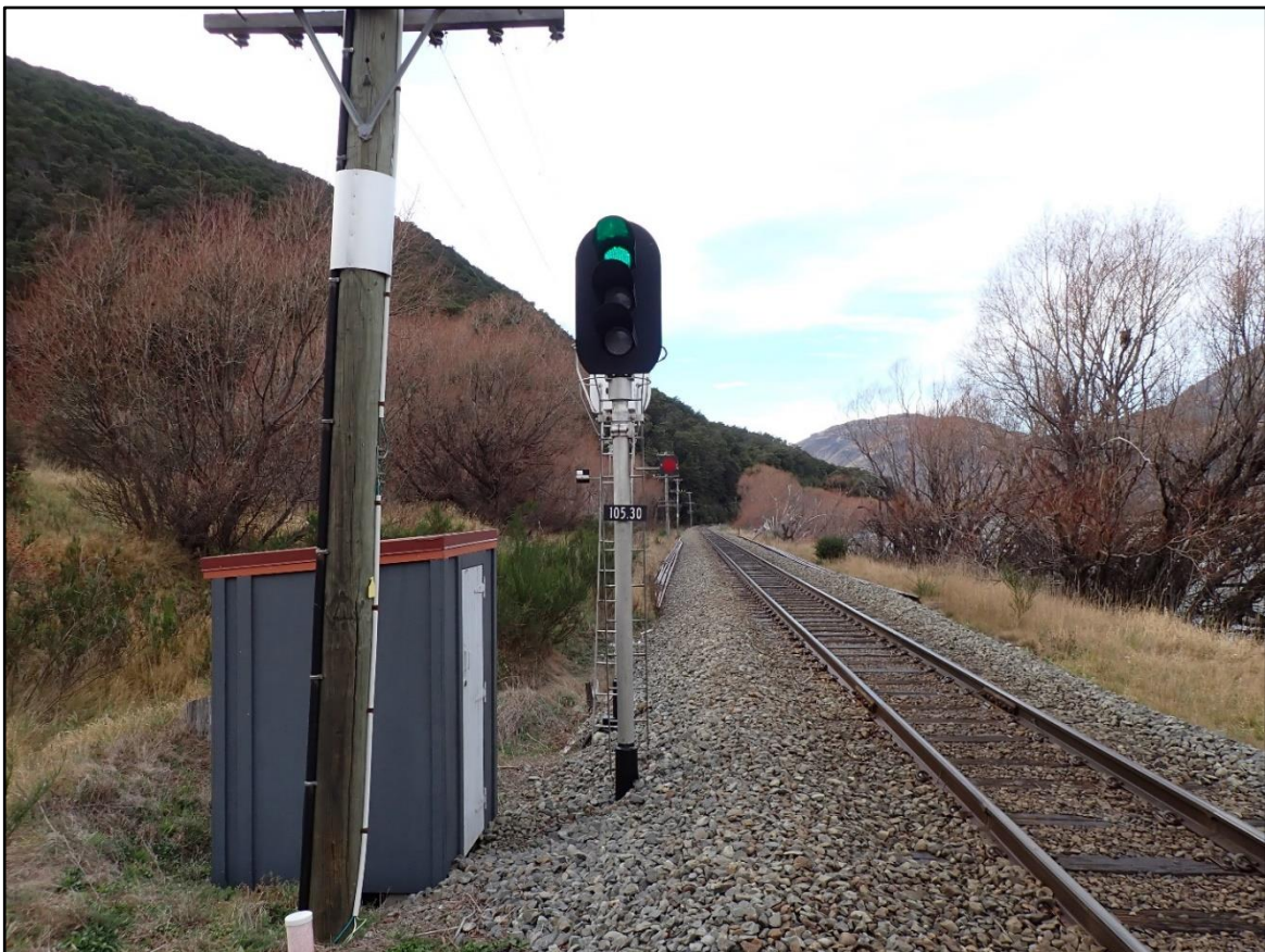
Figure 5: Intermediate signal 10530 (displayed yellow, not green, at the time of the incident)
