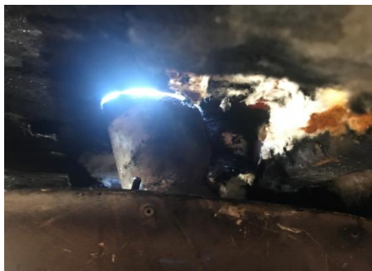
Figure 9: Daylight visible where exhaust tail pipe met ceiling of AG130
