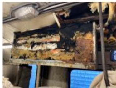
Photo 14. Exhaust silencer enclosure AG130. Part of IMG_2939.jpg
