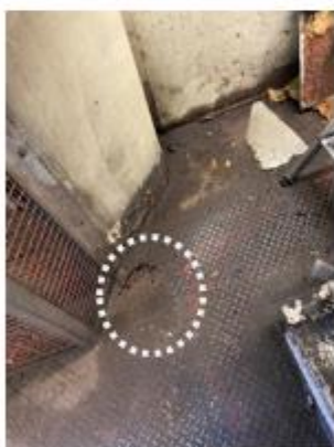
Photo 22 Floor of AG130 adjacent to the genset. White circle indicates rust area. IMG_2970.jpg
