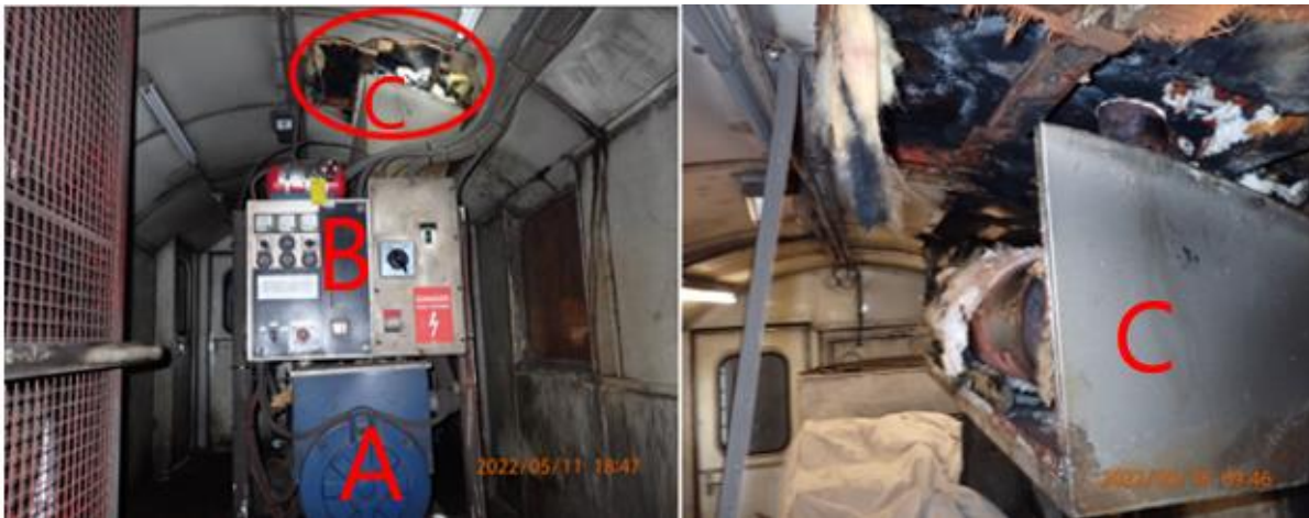
Figure 8: The AG130 auxiliary generator set after the incident
