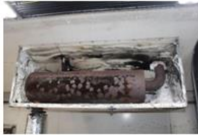
Photo 13. Part of the insulation removed from the exhaust silencer enclosure removed from AG176. IMG_2117.jpg
