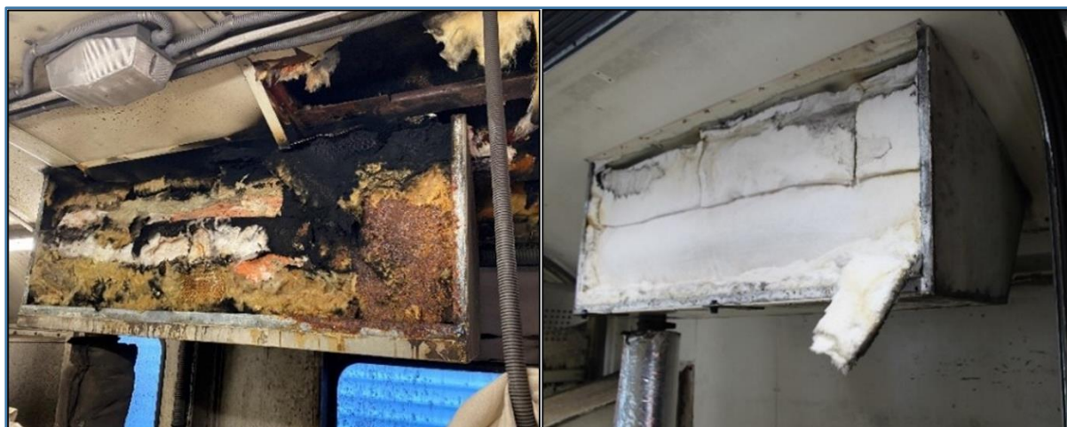
Figure 7: Top boxes of AG130 (left) and AG176 (right) showing condition of insulation (Credit: Fire and Emergency New Zealand)
