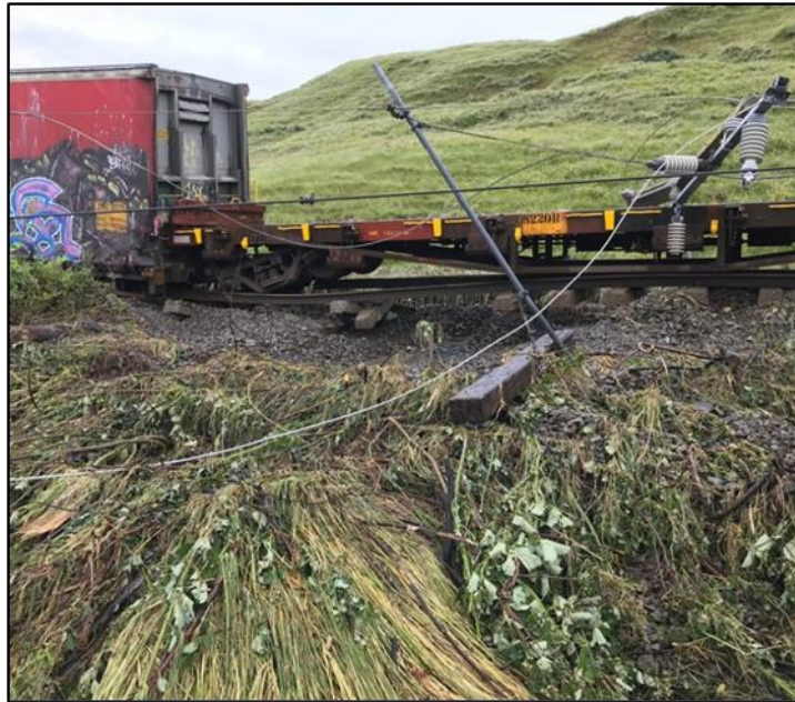
Figure 9: Washout showing unsupported rail (Credit: KiwiRail)
