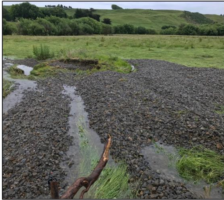
Figure 8: Ballast washed to western side of railway track (Credit: KiwiRail)
