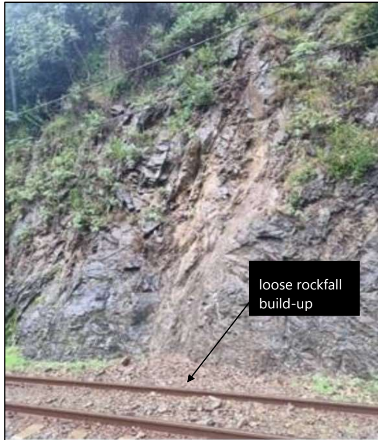
Figure 4: Rockfall site at the 3.567 km mark
