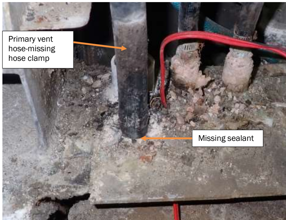
Figure 6: Primary vent hose connection to fuel tank (underneath the deck plate)
