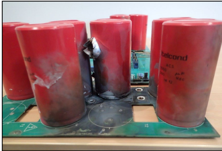
Figure 3: Failed capacitor from UPS A
