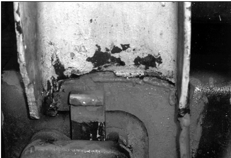
Figure 3 Closer view of the failed handgrip in position with previous weld repairs visible
