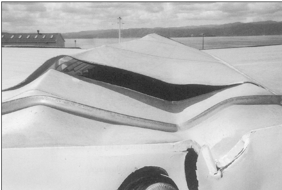
Photograph showing an outside view of the crumpled ceiling of the car deck
