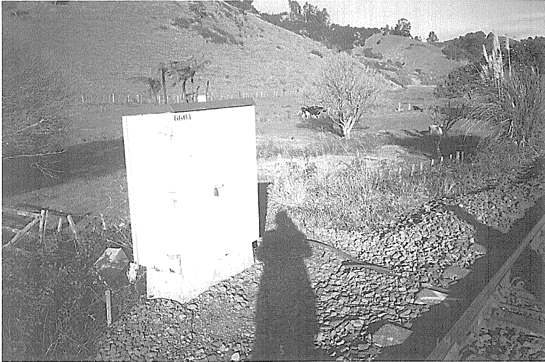
Figure 2 Signal location box 6617 (6603). General view looking south showing relativity to rail.
