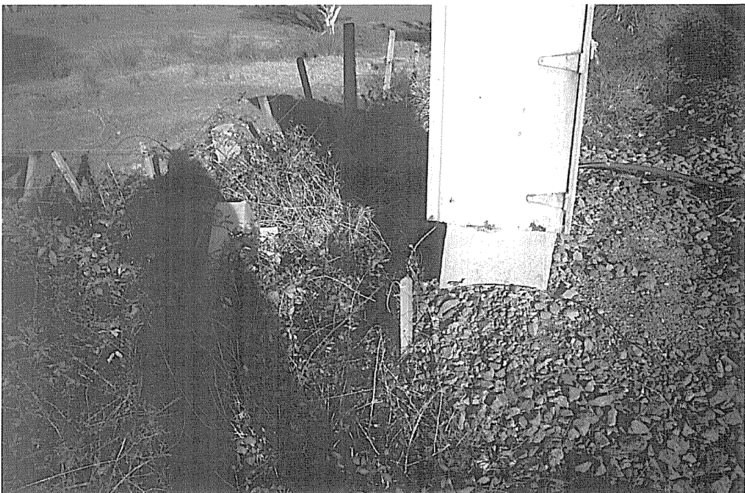
Figure 3 Signal location box 6617 (6003). View looking south showing earth wire at the north end and the rough terrain behind the box.
