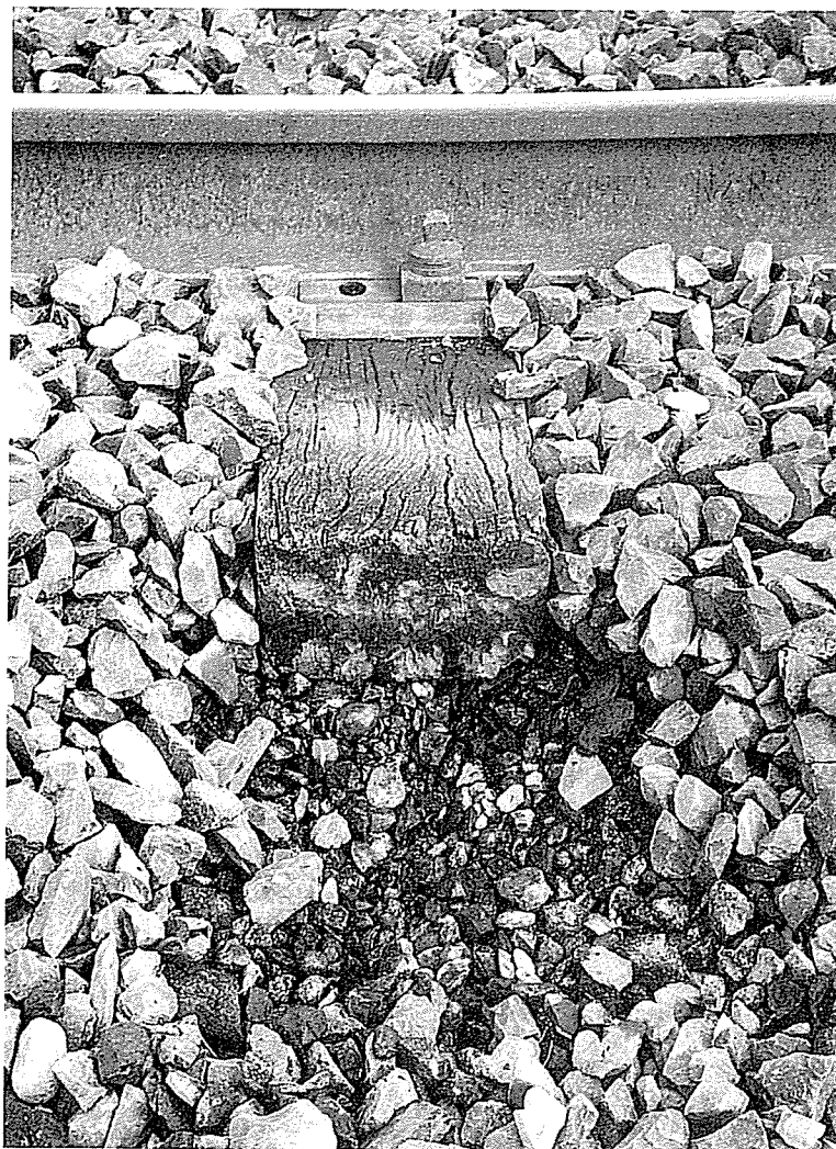
Fig 4: The careful removal of the ballast shoulder clearly reveals the difference between the top ballast and the small dirty material under the sleeper. At this location near the derailment site, the bottom ballast was wet, indicating a possible drainage problem.
