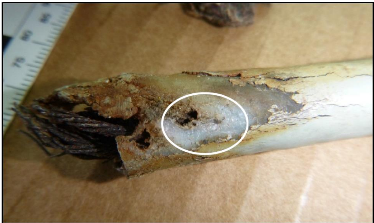
Figure 7 End of failed wire showing corrosion and sheath degradation
