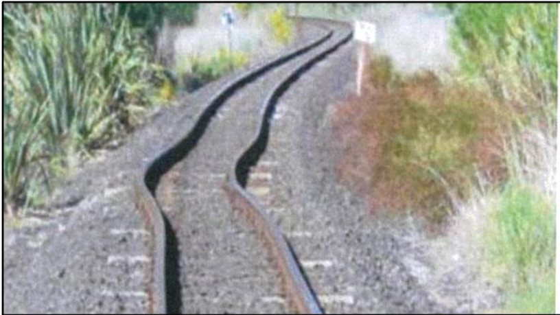
Figure 6 An example of a track buckle
