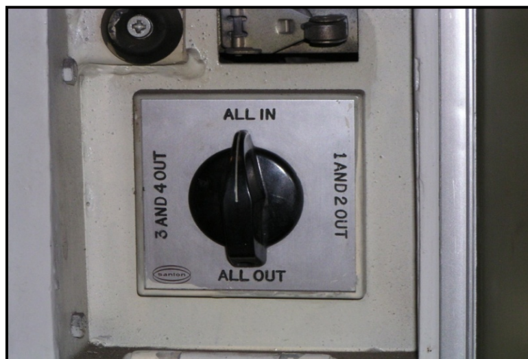
Figure 4 Traction motor cut out switch © Transport Accident Investigation Commission
