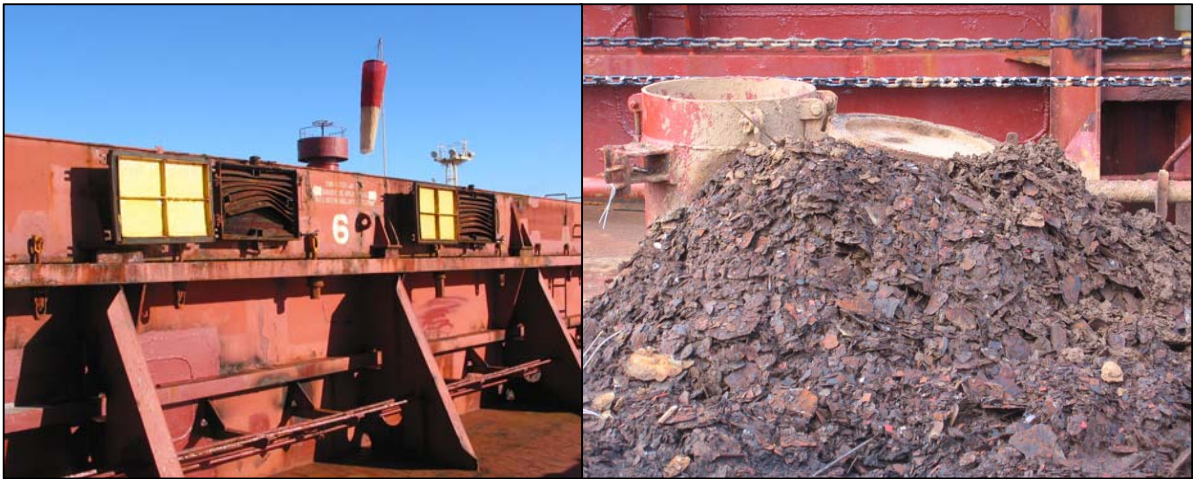
Figure 2 Damage to vents in number 6 hold and scale removed
