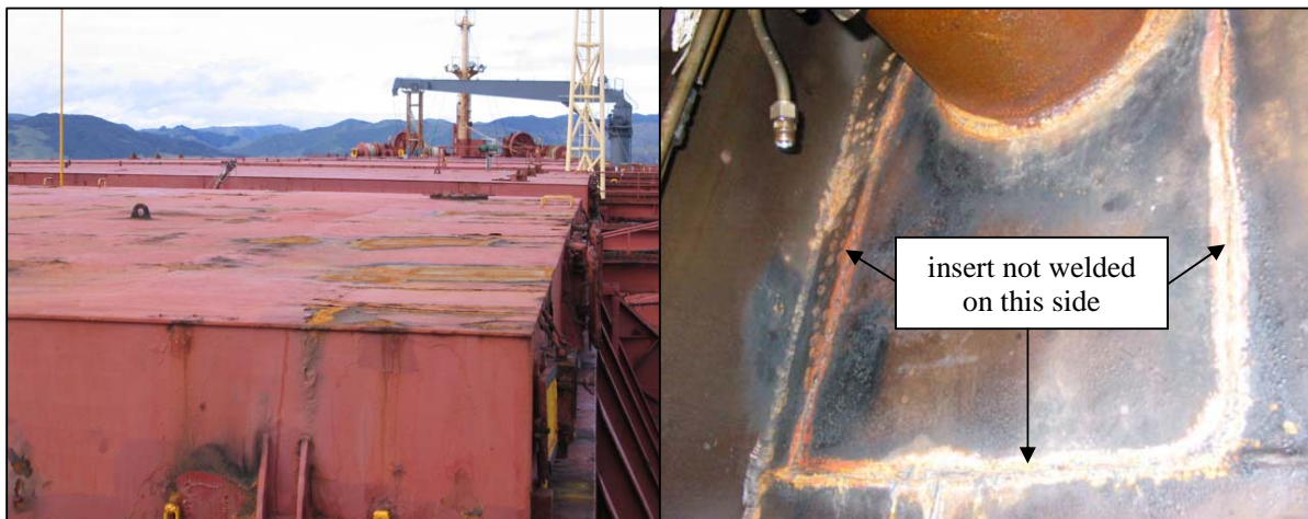
Figure 3 Deformed plates in hatch lid and insert in number 1 overflow recess
