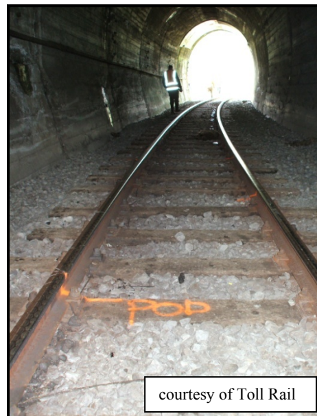
Figure 2 Track formation at the point of derailment
