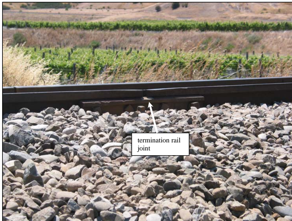
Figure 4 Batter and dip at termination joint; left-hand rail in direction of travel
