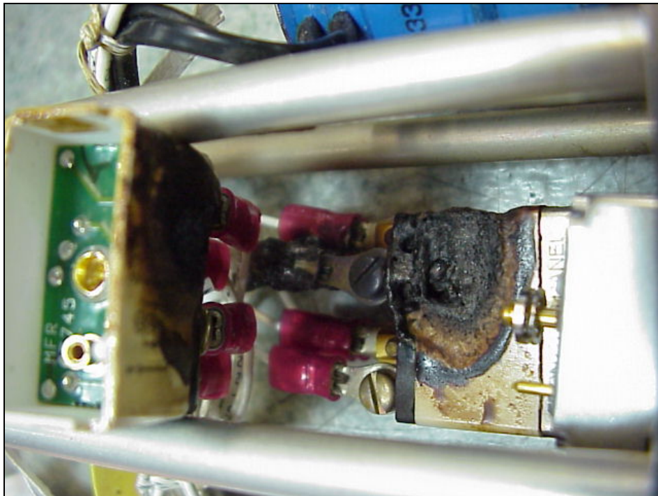
Figure 2 External burning of light switch assembly component
