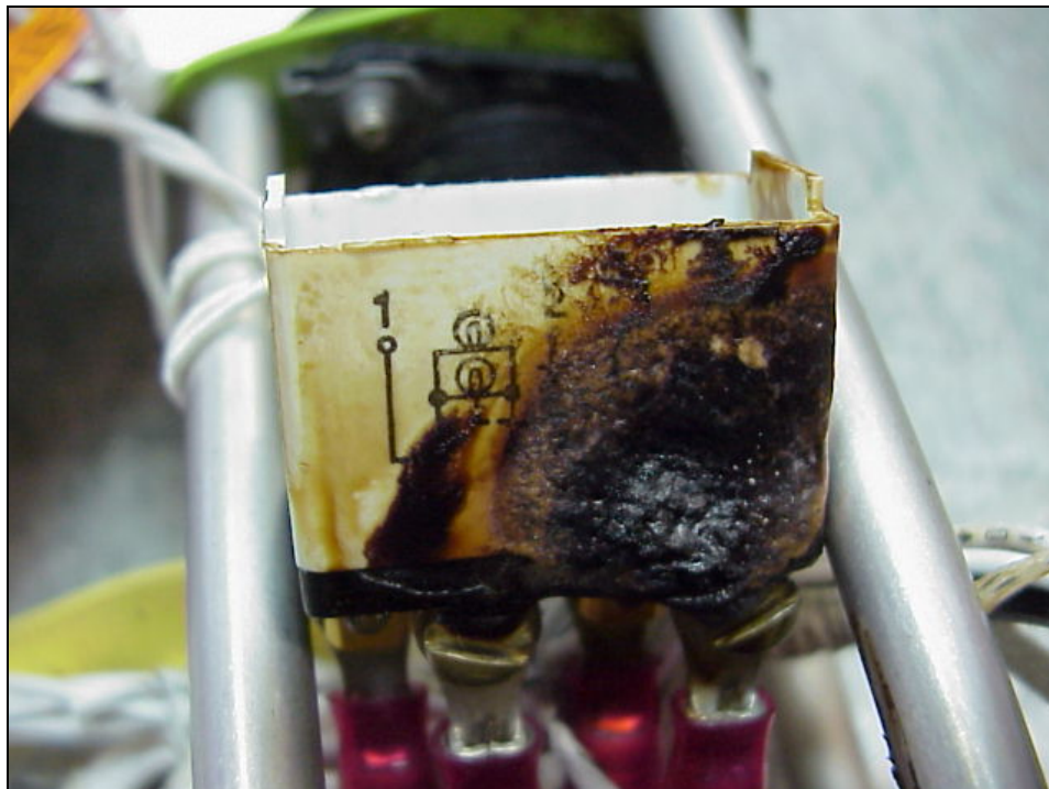
Figure 3 External burning of adjacent light switch assembly component
