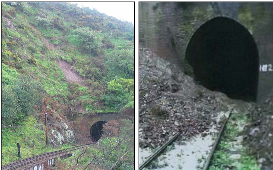
Figure 4 Developing landslide above Tunnel 2 (left) and debris blocking the track after sluicing (right)
