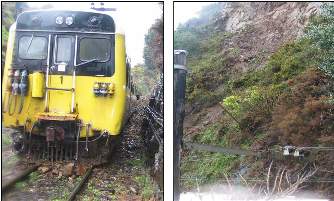
Figure 2 Derailed train (left) and origin of landslide debris from up hill face (right)
