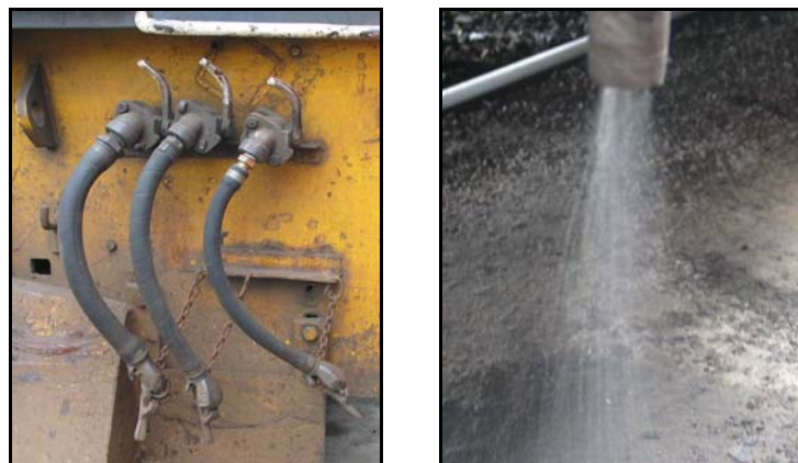
Figure 7 Headstock cocks, left, and condensation being expelled from a valve on right
