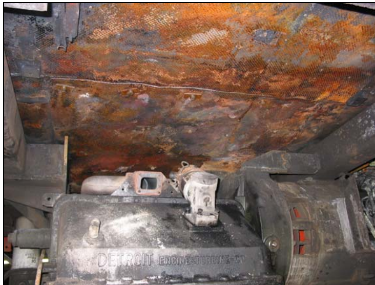
Figure 3 Damaged underfloor above the auxiliary motor
