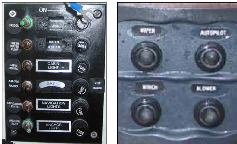
Figure 5 Switchboard located in the forward cabin and helm station switches
