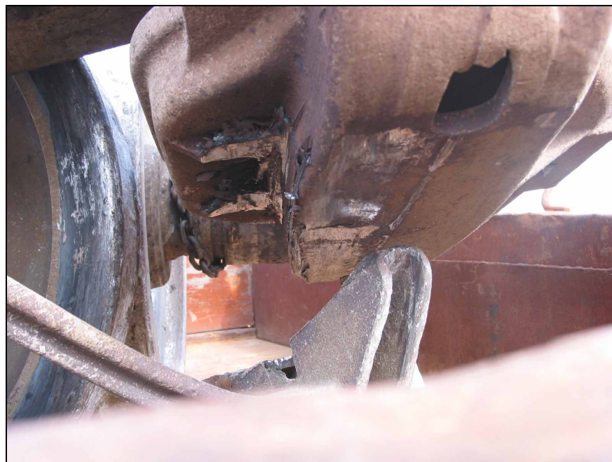
Figure 11 Worn away gussets
