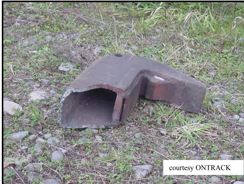
Figure 1 Fractured pedestal leg found trackside
