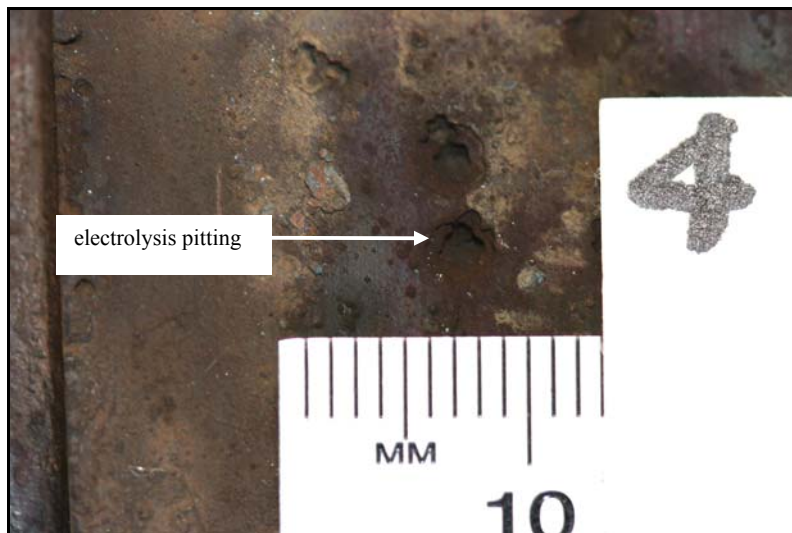
Figure 16 Electrolysis on liner of No. 4 cylinder
