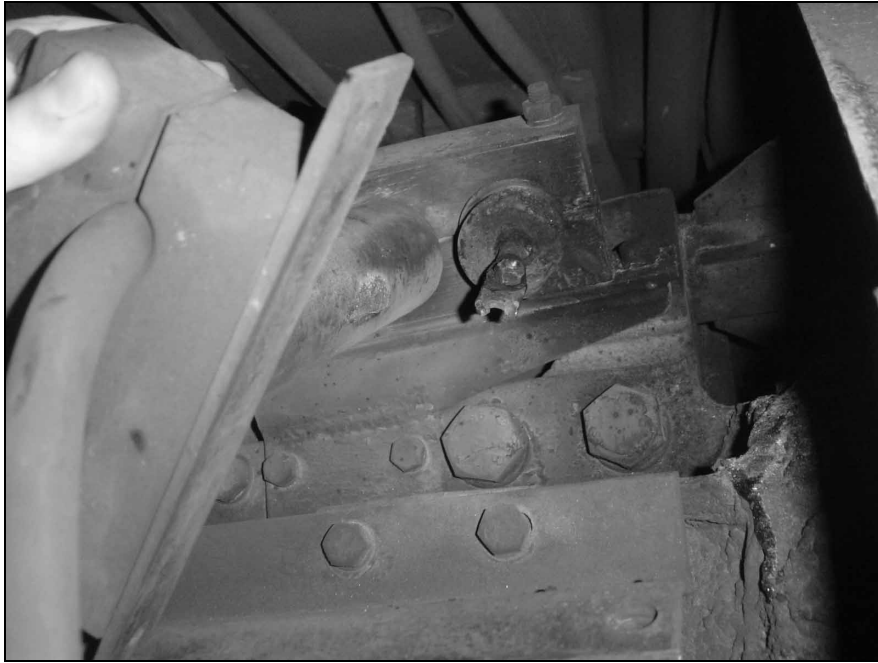
Figure 13 The cable clamp free to pivot and the failed crimp lug in the rear
