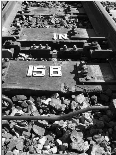
Figure 4 Sleeper damage at No 15 points
