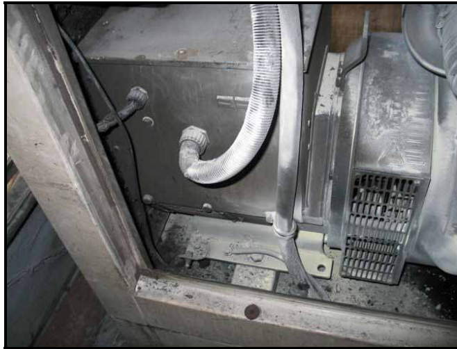
Figure 3 Alternator air intake and exhaust grill
