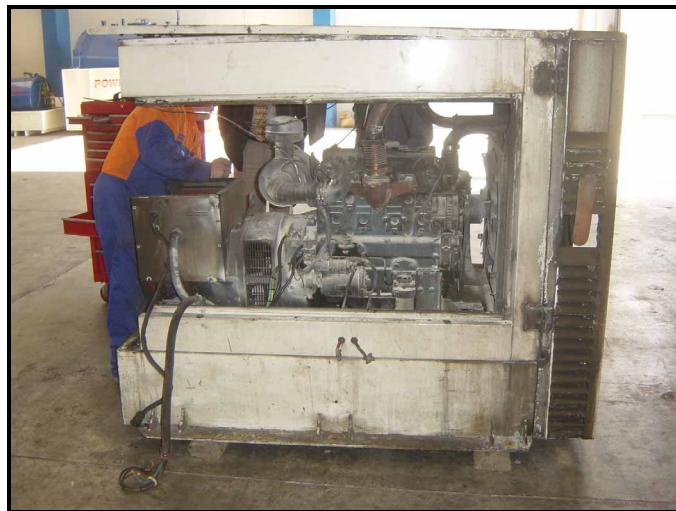
Figure 2 Generator enclosure with the side and front-end covers removed
