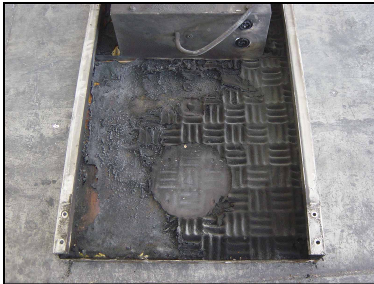
Figure 6 Burn marks to the soundproofing material
