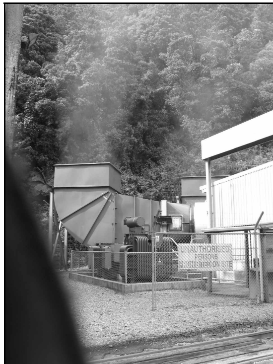
Figure 4 The extractor fan exhaust outlets at the western portal of Otira Tunnel
