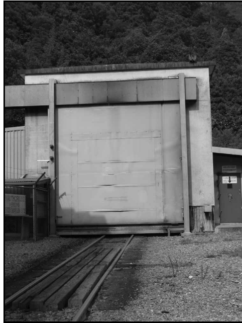
Figure 3 The sliding door in the closed position at the western portal of Otira Tunnel
