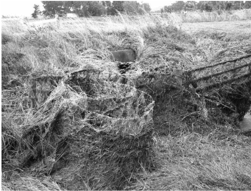
Figure 4 The fence in front of the farm culvert after the flooding
