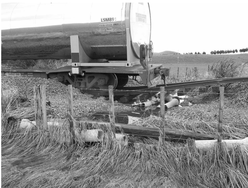
Figure 6 The downstream side of culvert 43.554 after the washout
