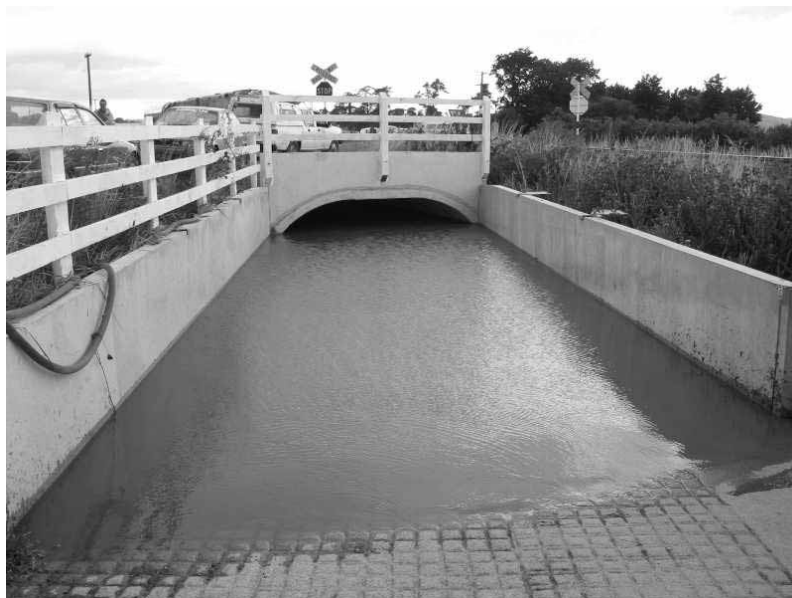
Figure 12 The southern end of the flooded stock underpass
