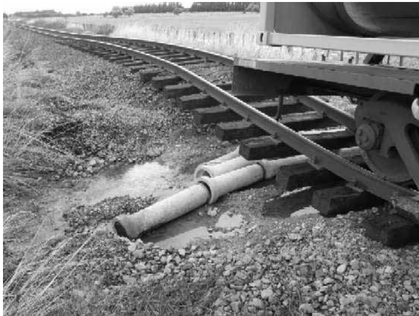
Figure 5 The upstream side of culvert 43.554 after the washout
