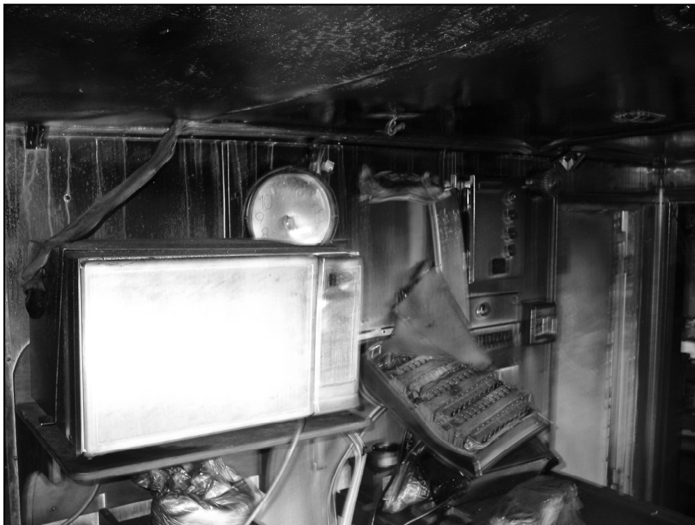
Figure 7 Forward bulkhead of the messroom showing microwave, melted clock and circuit breaker cabinet
