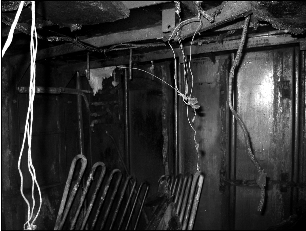
Figure 6 Refrigeration space showing fallen coils and hanging wires
