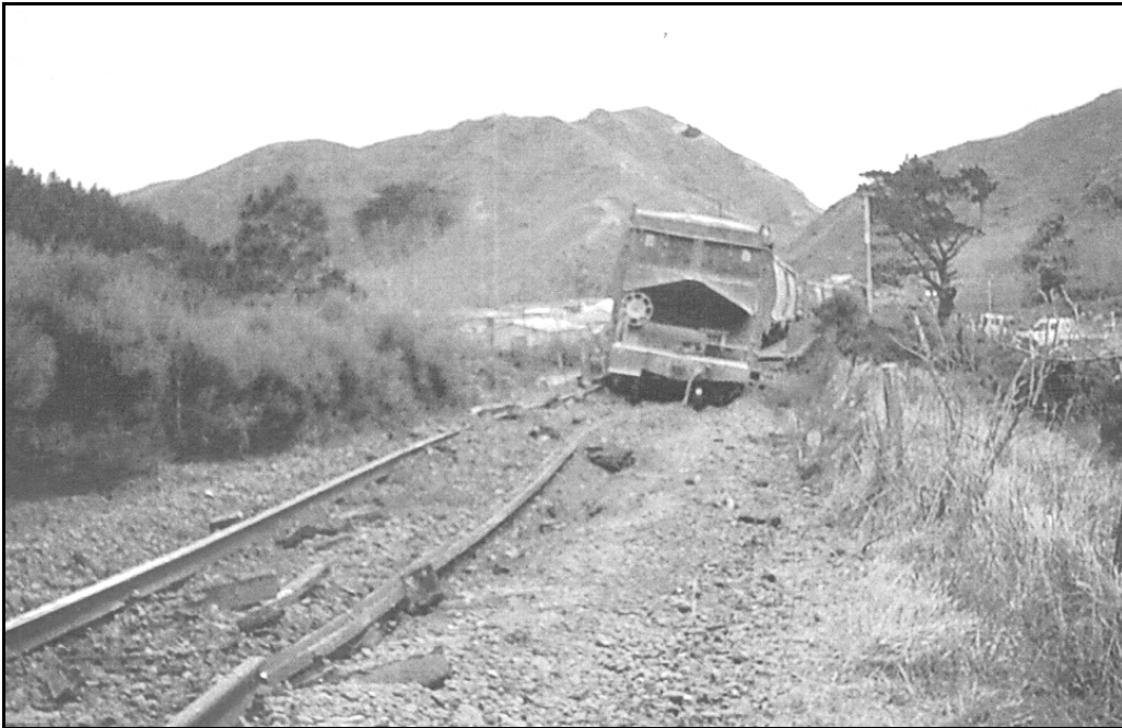
Figure 2 Damaged track past the POD
