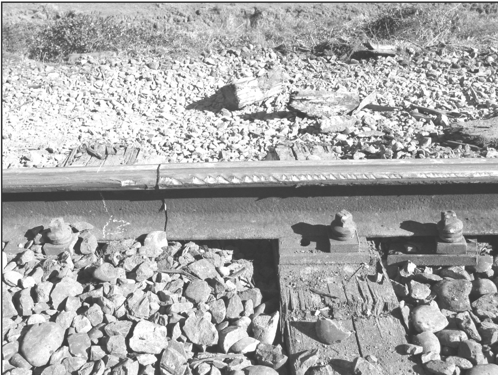
Figure 7 The fractured high leg rail with the heavy scoring visible
