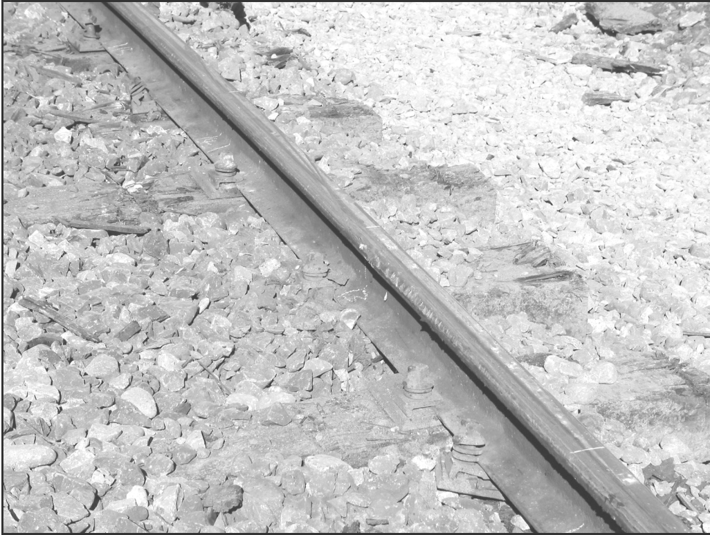
Figure 6 The heavy scoring on the gauge side of the high leg rail
