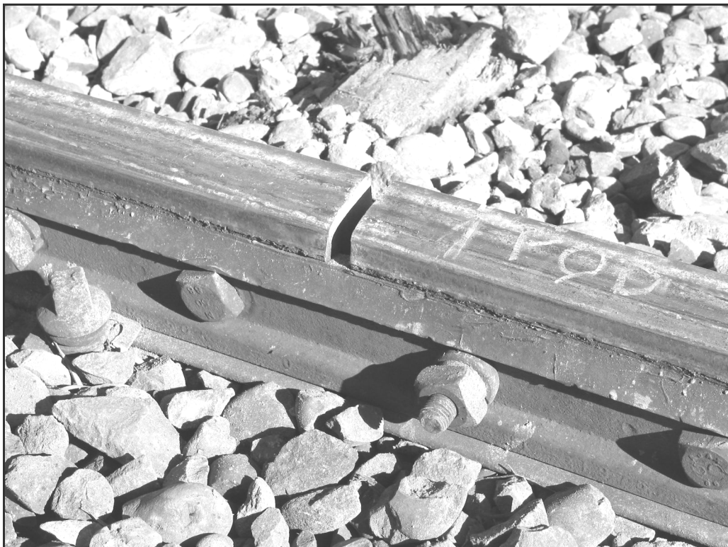
Figure 5 The marks at the point of derailment
