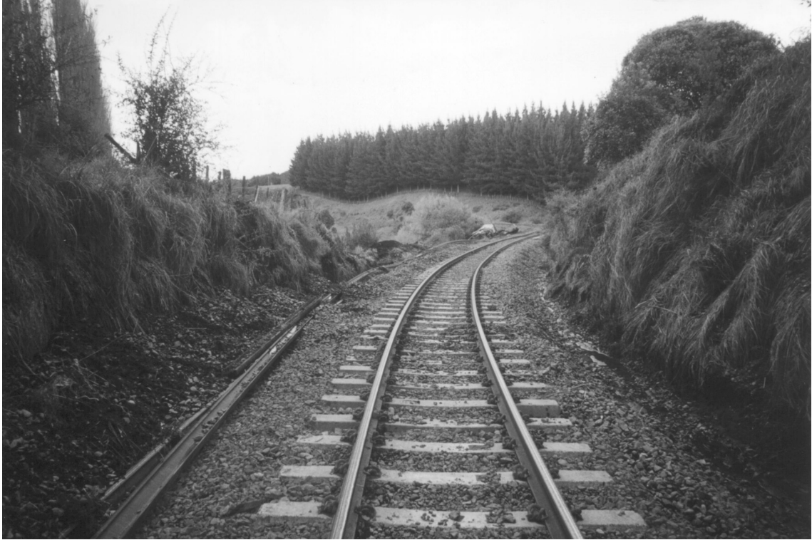
Figure 1 Looking south from the POD at the derailed locomotives in the background
