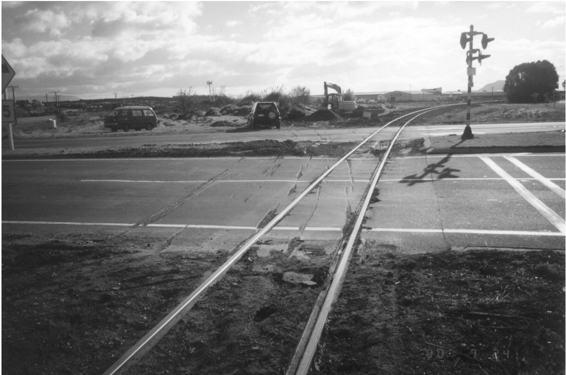
Figure 4 Wheel marks of derailed DC 4749 crossing SH 2 (looking in direction of travel)
